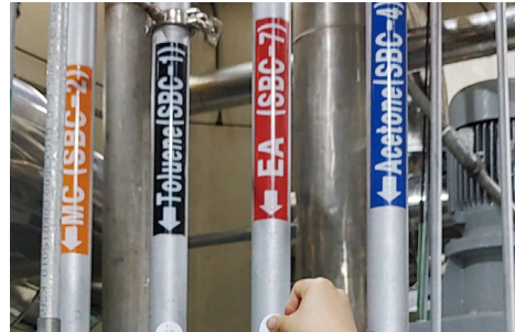
Labeling of hazardous chemical pipelines
